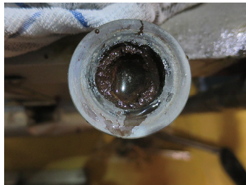
Fig. 1. Blocked cooling water piping for the turbines.
