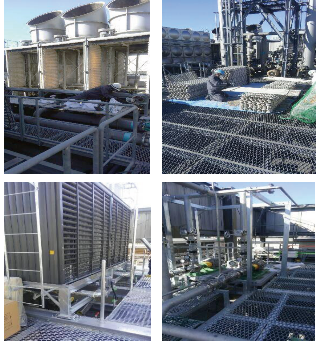
Fig. 1. Photographs of the four systems of RIBF cooling tower overhaul and new cooling systems for RILAC's superconductive.
