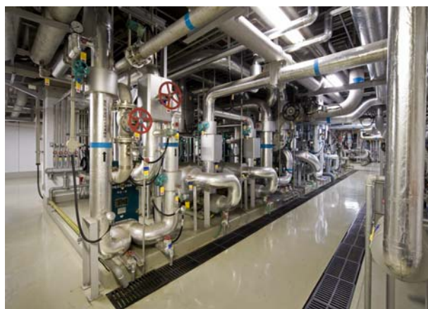
Fig. 3. Photograph of the Cooling water-pump on the first floor.
