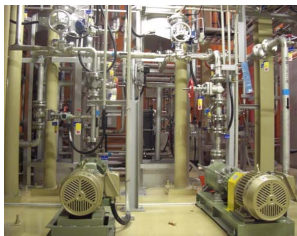
Fig.4. The Sub-system cooling pump. (IRC room on the second floor in the basement)
