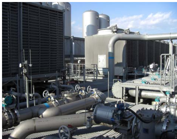
Fig. 2. Photograph of the Cooling Towers on the rooftop.
